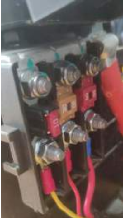
Fuse is located under the positive terminal of the battery.
